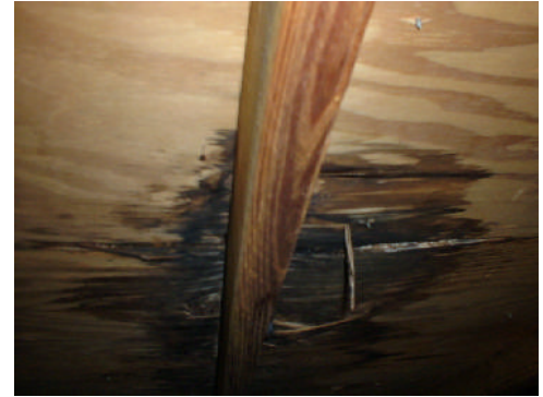
Photo # 5 ROOF LEAK AS OBSERVED FROM ATTIC
